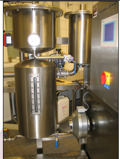
Dichlormethane (DCM) – Recycling Unit with condenser and storage tank of reusable DCM.
