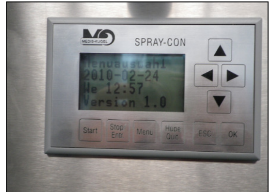
SprayCon contro unit with display and visual and acoustic alarm. All messages in english language.
